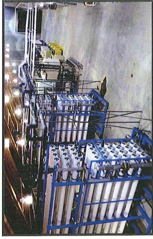
Colorado River MWD – Big Spring Raw Water Production Facility
